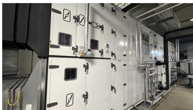
(b) Central air handling unit in the test hall
