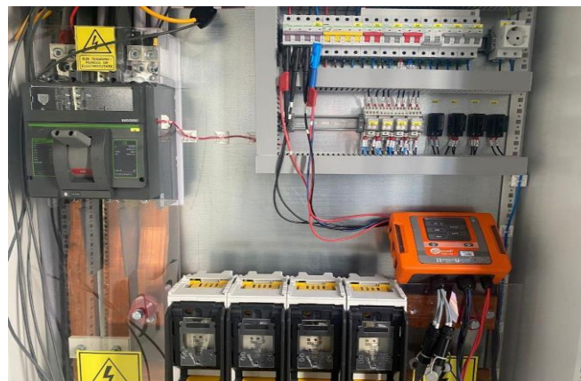
Figure. 3. General 0.4kV switchboard of the PV plant where the network analyser was installed
